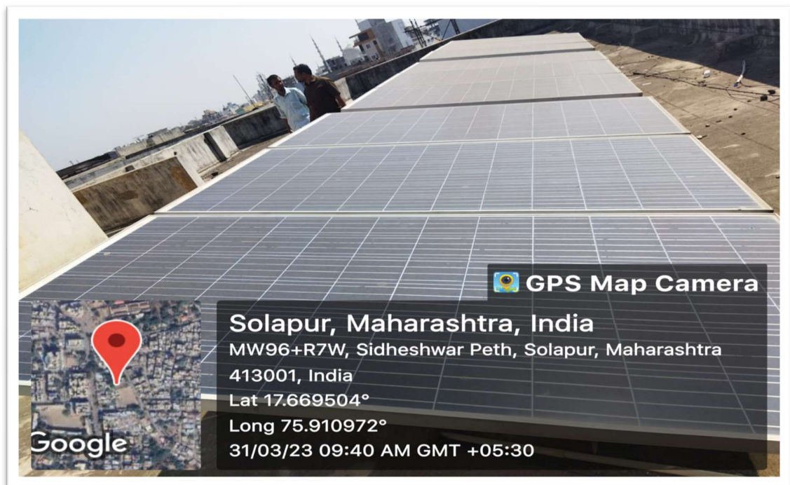
Fig.38: Solar Panels on the College Building Roof
