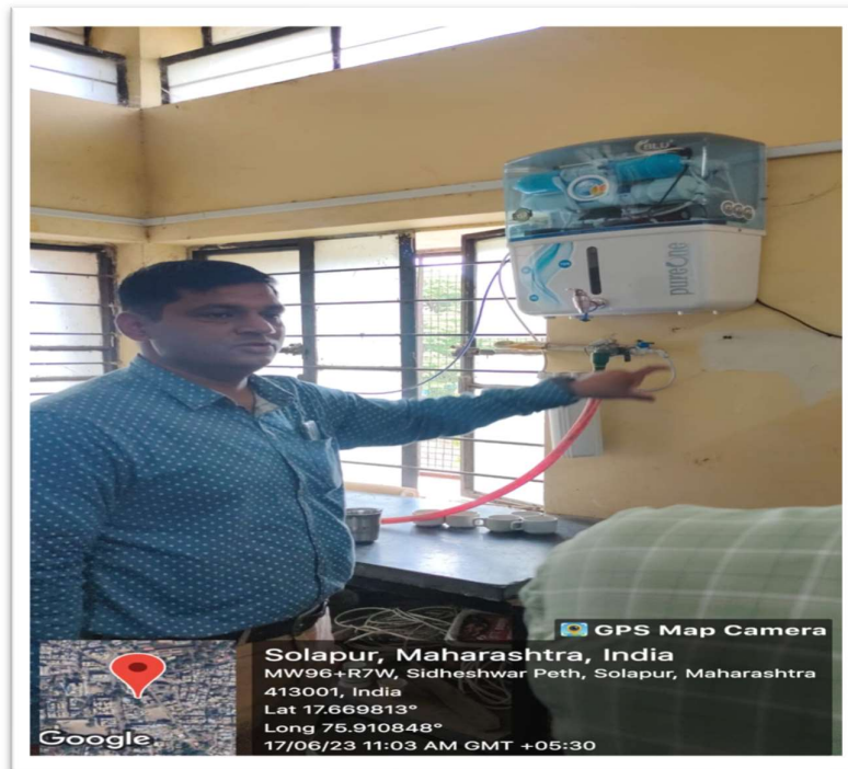
Fig.31: RO Water plant a,b,c,d
